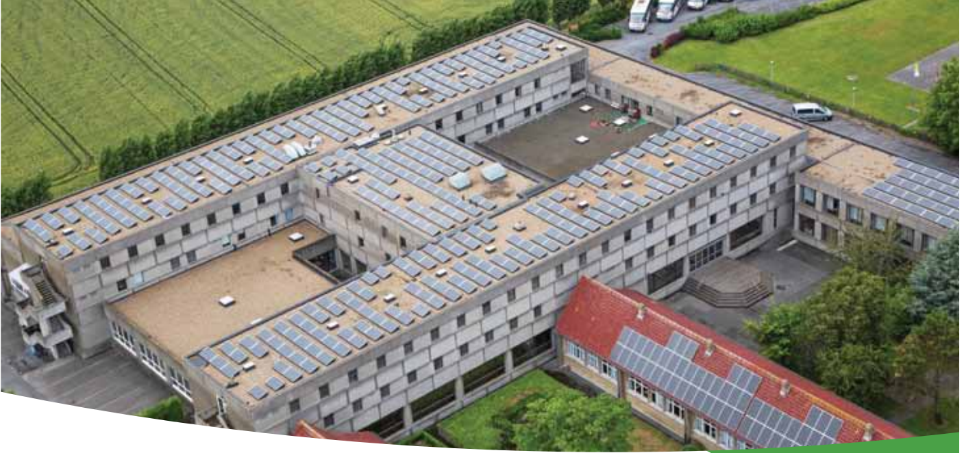
Solar panels on roof of office buildings
